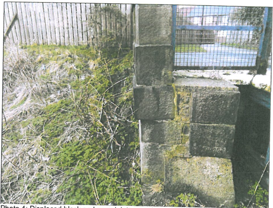
Photo 4: Displaced block and open joints over the south abutment
