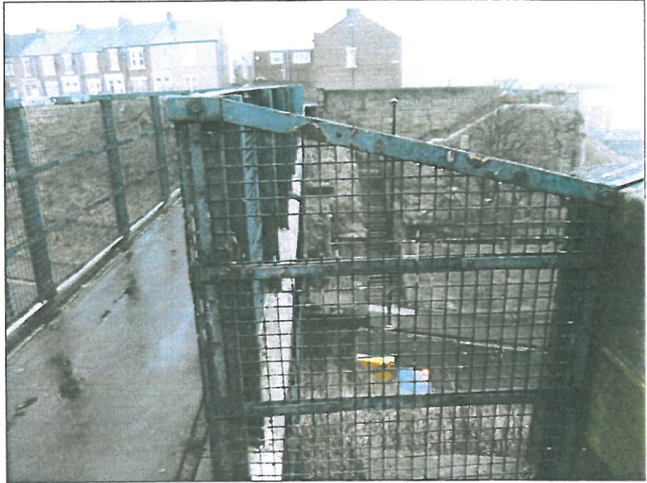
Photo 25: General paint failure and associated corrosion to parapet members
