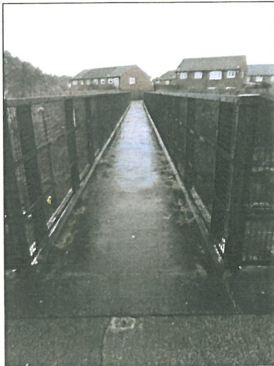
Photo 26: View of footbridge surfacing showing vegetation at the edges of footway
