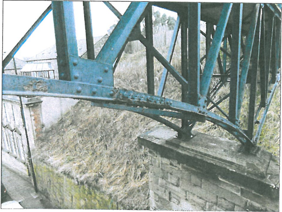
Photo 15: Paint failure and associated corrosion at splice connection
