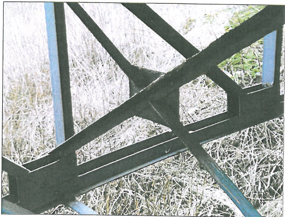
Photo 16: Paint failure and associated corrosion on the bracing members
