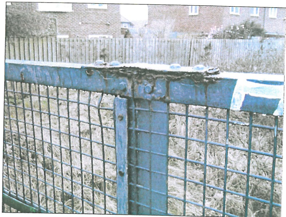
Photo 24: Paint failure and steel flaking at top of parapet – typical for few locations
