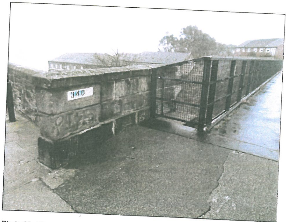
Photo 28: Minor pointing loss over the approach parapets
