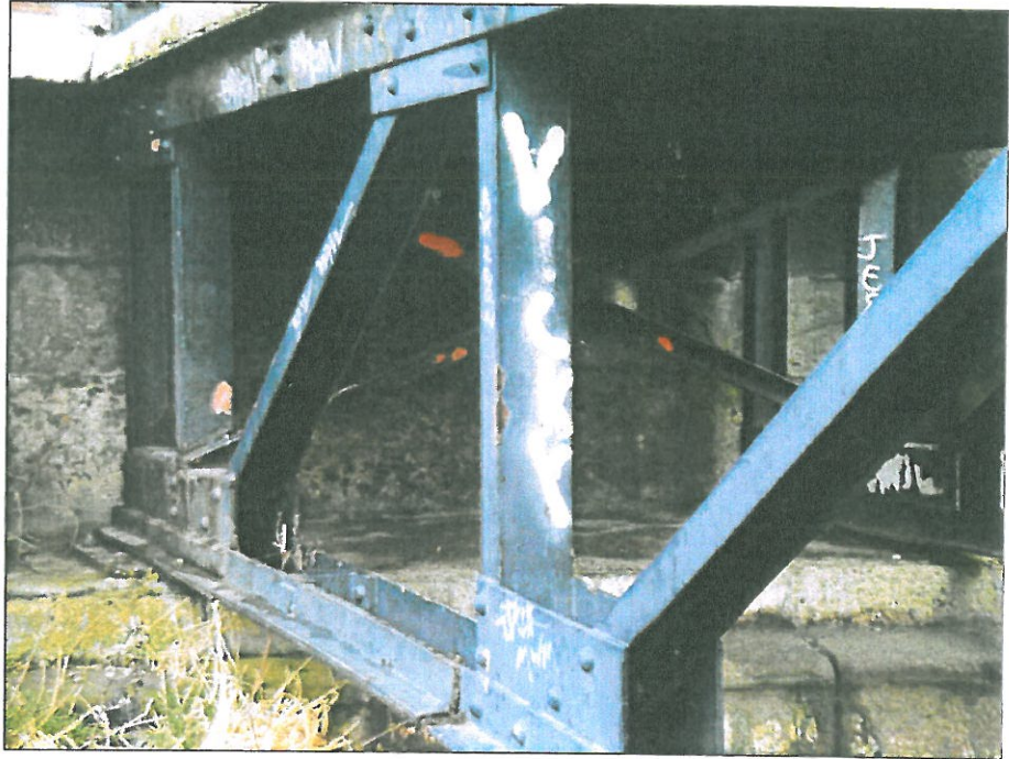
Photo 17: Graffiti on superstructure members
