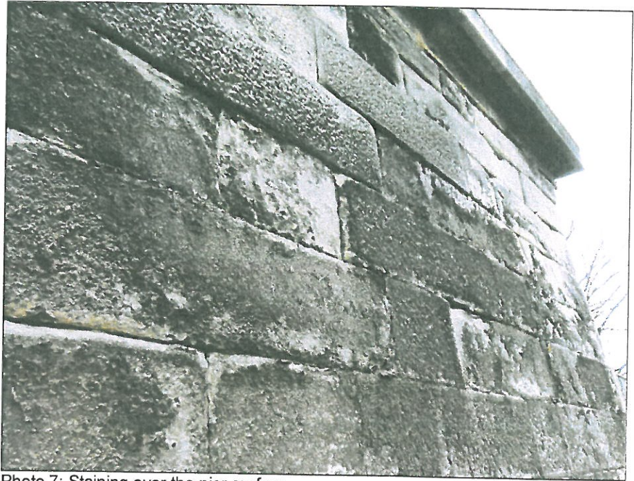
Photo 7: Staining over the pier surface
