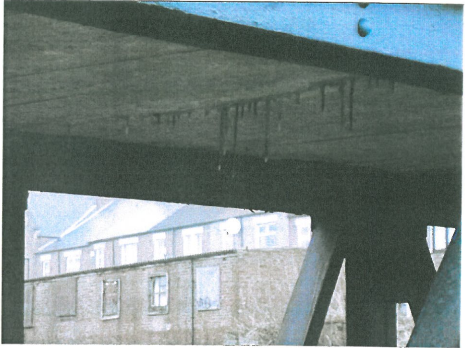
Photo 21: Accumulation of leaching salts on the deck soffit - typical
