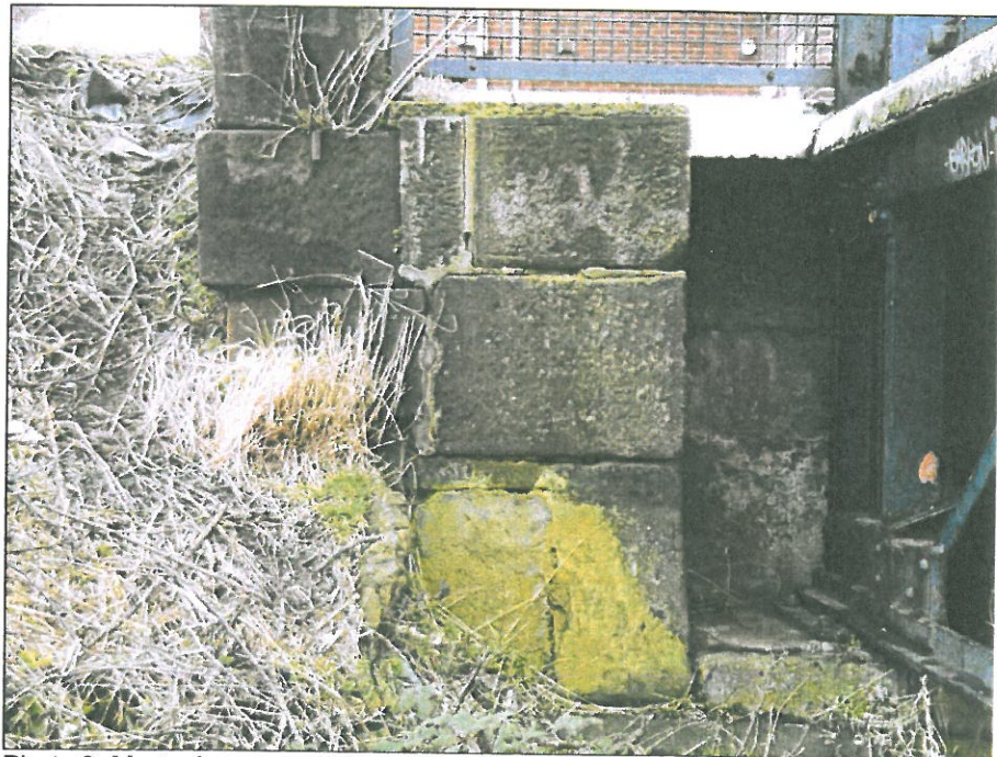
Photo 2: Mortar loss, open joints and algal staining at north abutment
