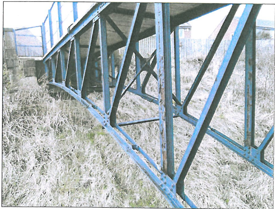
Photo 12: View showing paint failure and associated corrosion on the superstructure
