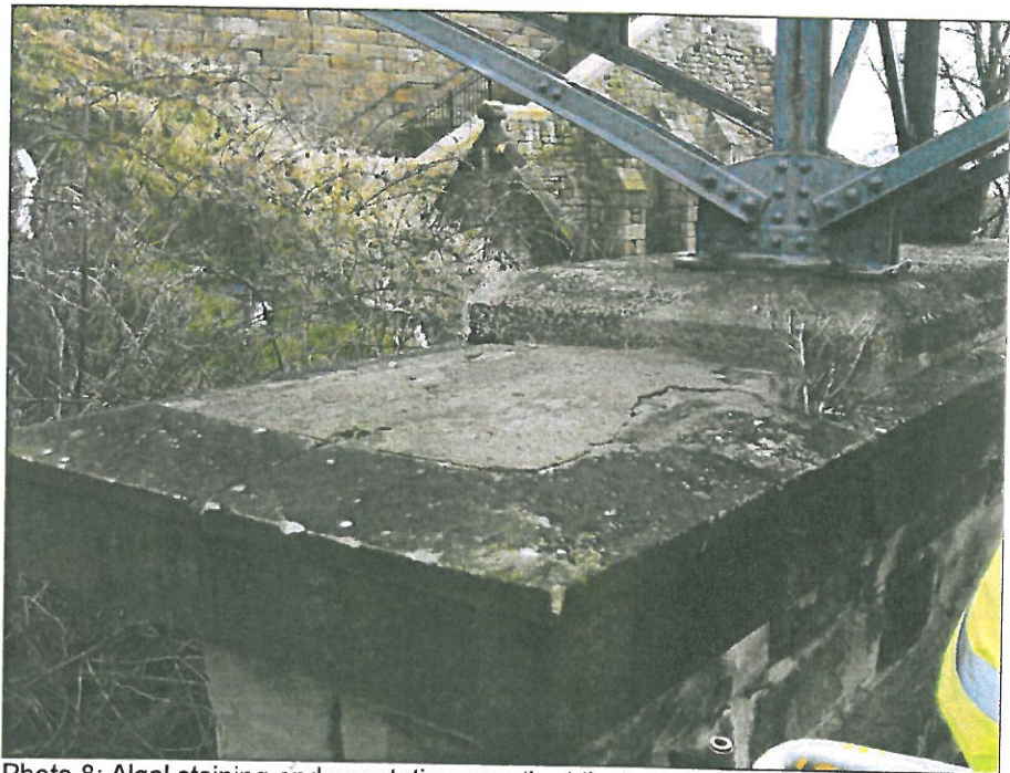
Photo 8: Algal staining and vegetation growth at the top of north pier
