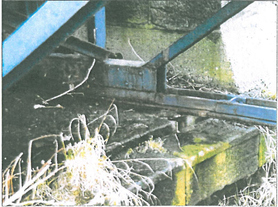
Photo 29: Corroded bearing plate under the longitudinal steel members
