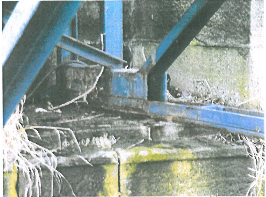
Photo 19: Corrosion to steel members over the abutment connection – typical
