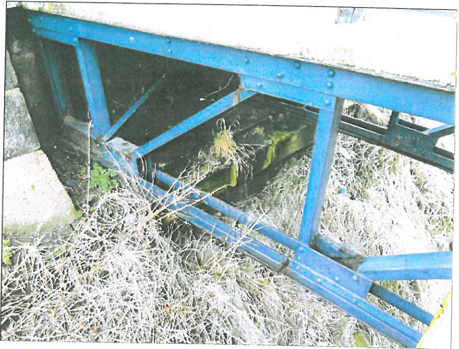
Photo 3: Algal staining and vegetation growth to the south abutment bearing shelf
