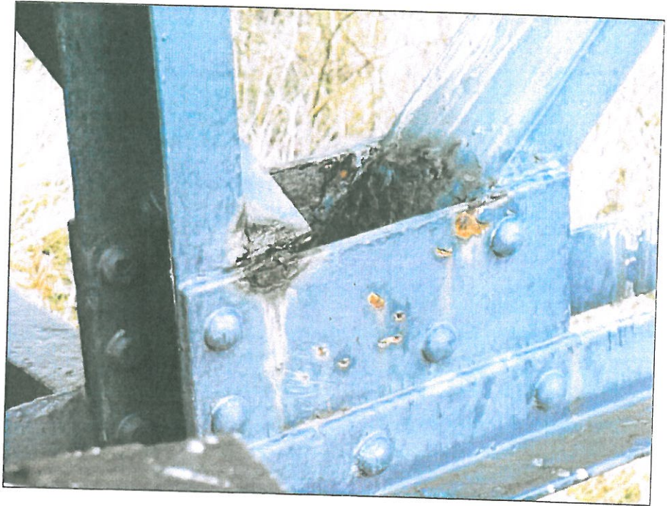
Photo 13: Paint failure and associated corrosion at the connection – typical
