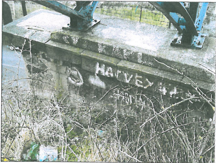
Photo 11: Graffiti at the pier elements
