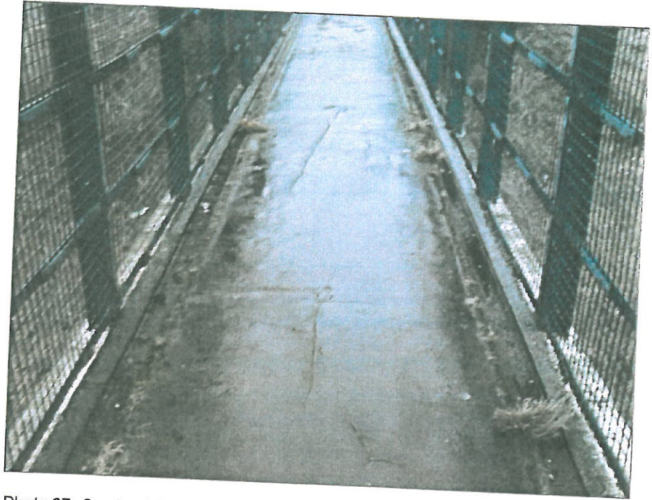
Photo 27: Cracks visible on the top of surfacing
