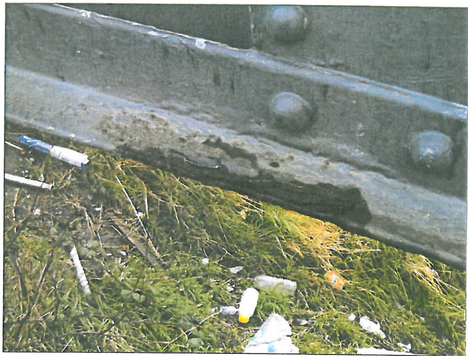
Photo 18: Steel flaking at the steel member
