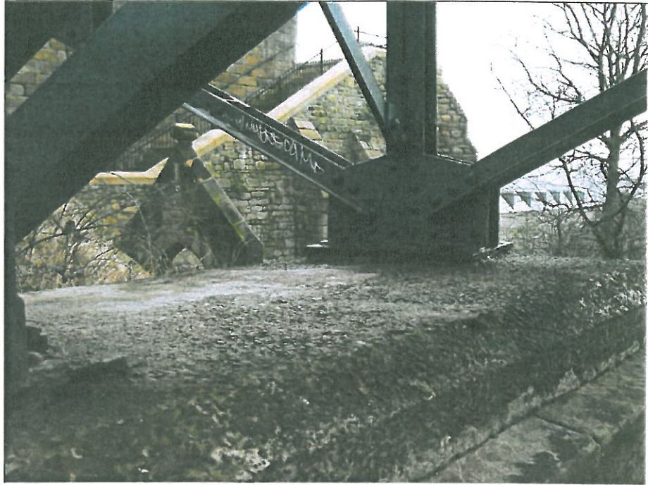
Photo 9: Scaling at the bearing plinth over the northern pier
