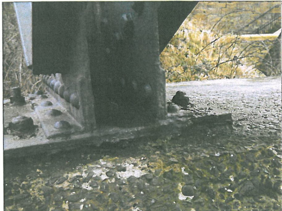
Photo 20: Corrosion and steel flaking at the pier connection – typical
