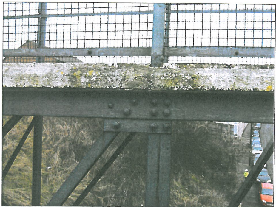
Photo 22: Algal staining and honey combing over the deck edges
